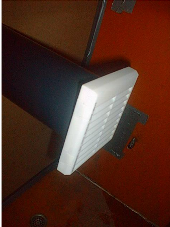
Figure 1. The indoor end of the duct with louvred ventilator plate fitted.
