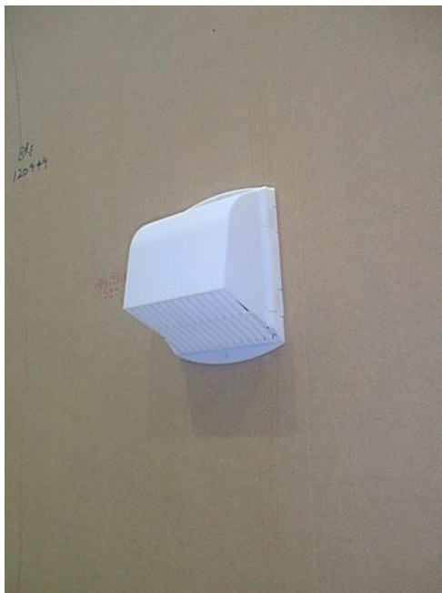
Figure 2. The outdoor end of the duct with cowl fitted
